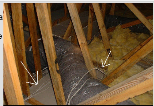
Insulation missing over kitchen ceiling
