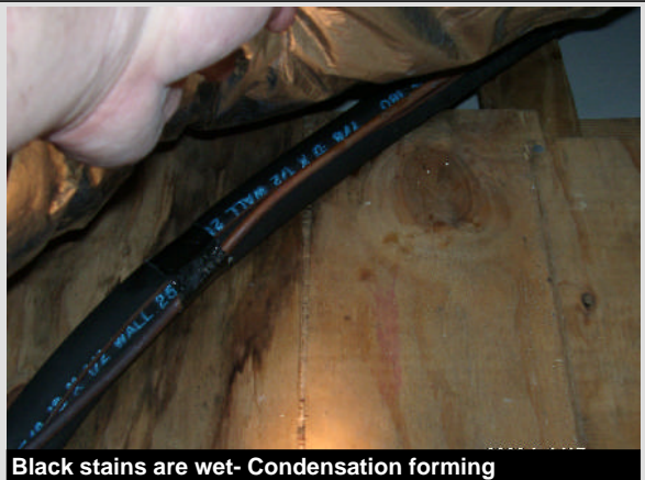
Black stains are wet- Condensation forming
