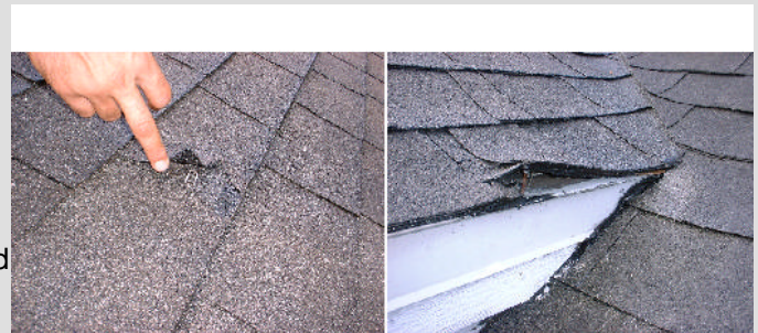
Protruding staple - Uplifted edge flashing
