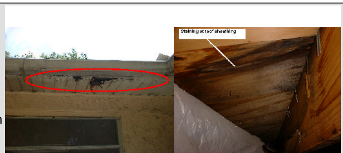
Damaged Overhang/Roof Problems/Leakage
